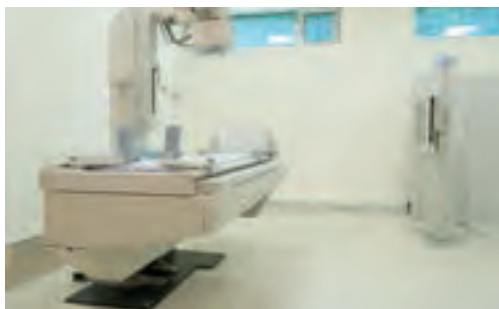
Radiography & fluoroscopy examinations are performed on the Toshiba Raffine remote controlled digital RF system with integrated FPD and a portable FPD in the vertical Bucky stand
