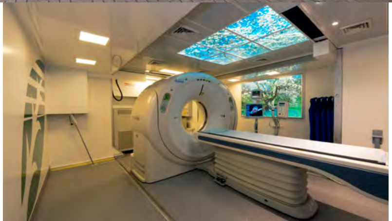
Mobile CT system and soothing scenes on the ceiling and side wall.
